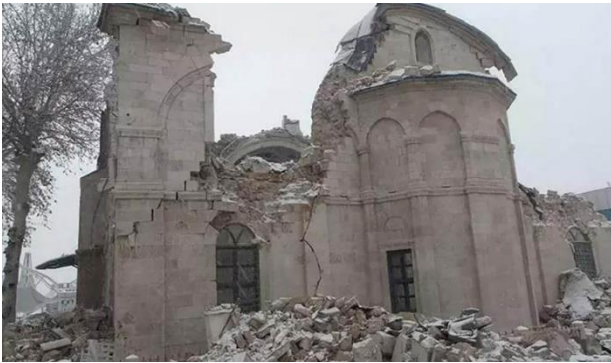
Fig. 5 Ulu Mosque after earthquake, Kahramanmaraş [16].
