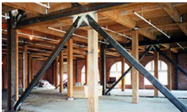
Fig. 7 Seismic retrofitting of a soft story, San Francisco [21].
