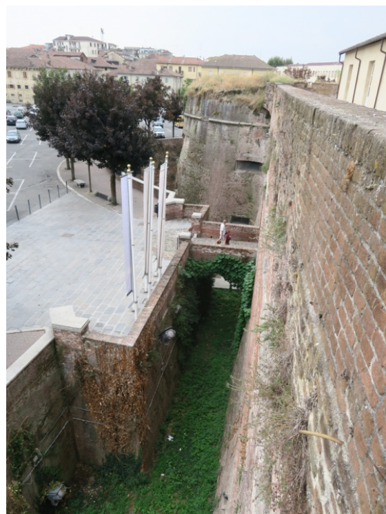
Fig. 1 View from the north of the south-east bastion, of the eastern curtain and of the counterscarp of the moat.
