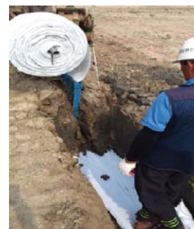
Fig. 5 Test construction of subsurface irrigation and drainage using non-excavation single pipe method.
